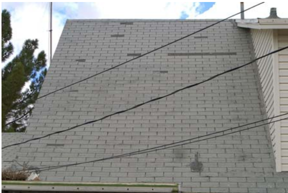
Multiple shingles missing from this area.
