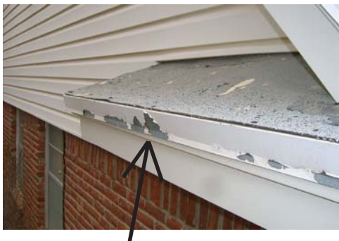
Paint peeling from the flashing all around the house.
