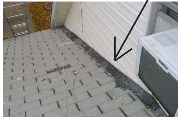
Some shingles missing from this area also.
