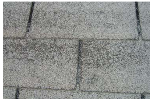
Shingles are showing their age when the aggregate is missing.
