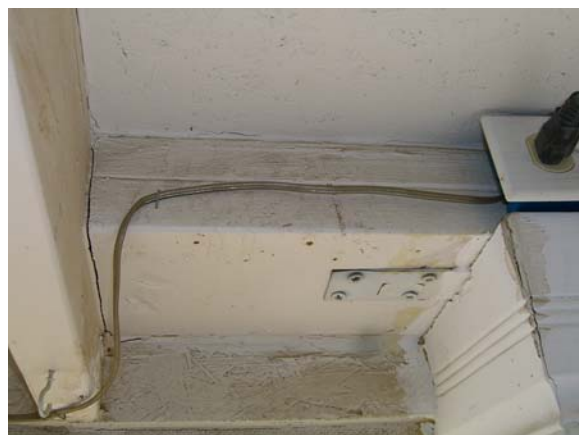
This wire to the outside outlet is unprotected and is the incorrect wire that you can use for this application.
