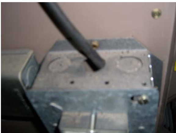
This wire to the junction box for the furnace is going through that should be grommet protected
