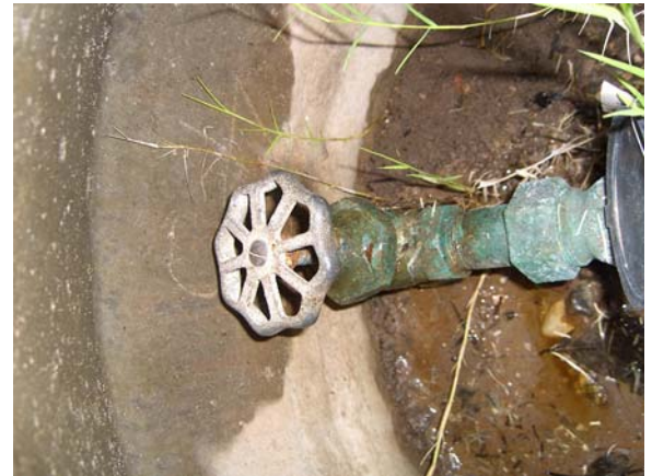
Small leak on city side of meter.
