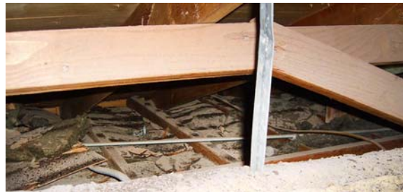
Even if you do not add blown insulation, you should repair these areas that do not have any insulation.
