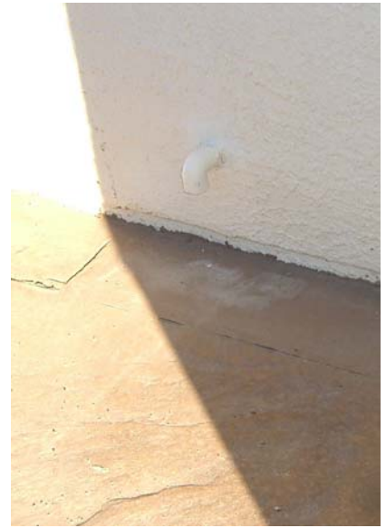
A/C condensate line will make a mess in this area.
