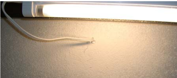
Electric cord going through the wall.
