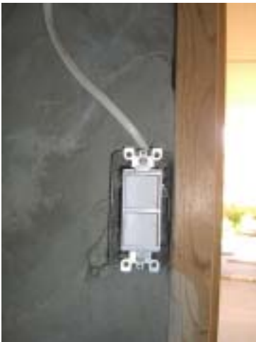
On the left is a switch that does not have a cover plate.
