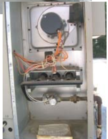
This is your unit on the roof with the cover removed. The unit appears clean.
