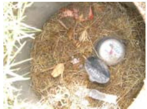
Water vault needs cleaning out
