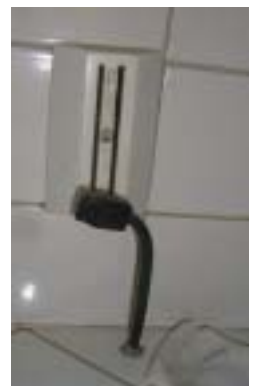
This cord should be in a conduit to protect it and to prevent a fire hazard.
