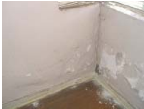
Damage on front bedroom wall
