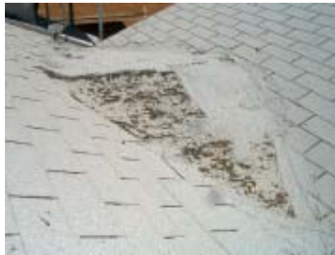
Another area not replaced with the new roof and is in very poor condition.
