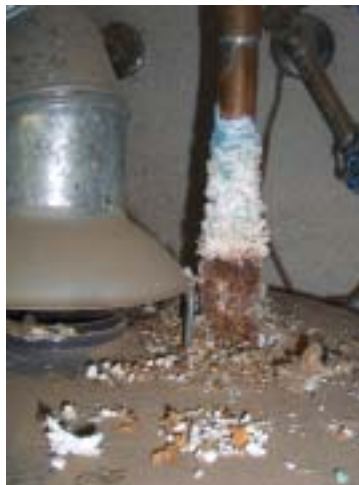
Corroded pipe has stopped the leak for now
