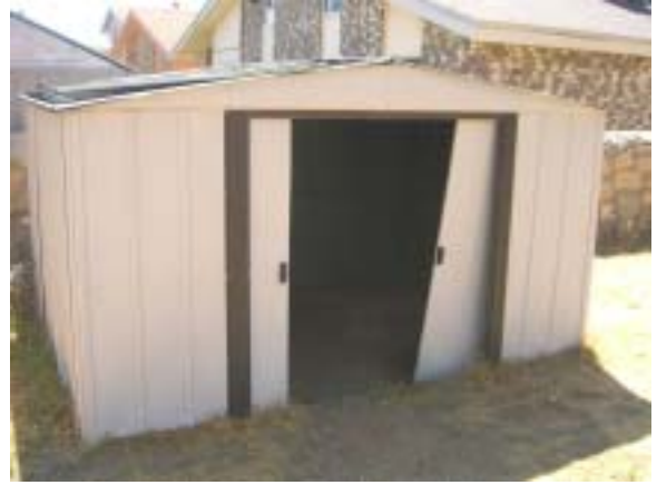
The shed is in bad shape. There is no foundation - it is just sitting on the ground.
