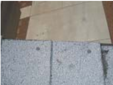
Here is the photo showing a sample area of exposed nail heads.
