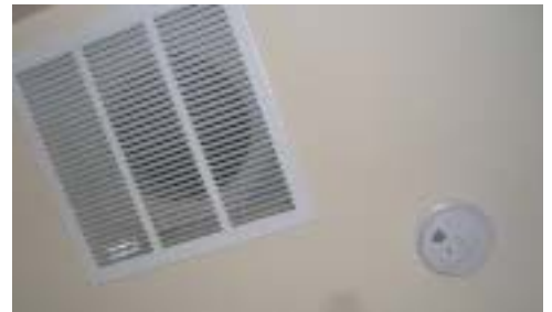
Vent too close to alarm
