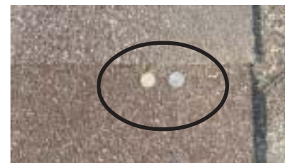
Example of exposed nail heads
