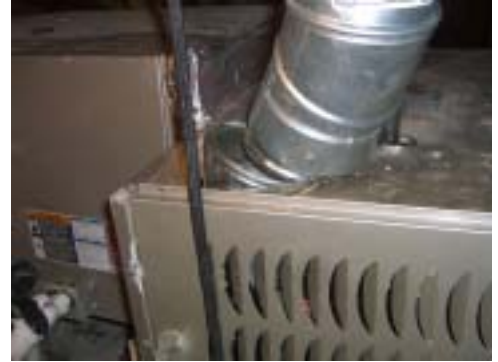
Flue pipe not properly connected.
